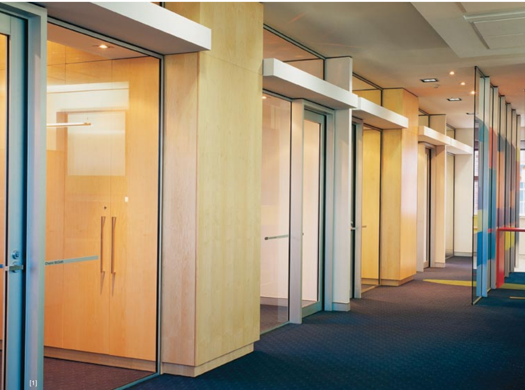
Above [1] ... Schiavello fitout works feature custom built joinery, partitioning, bulkhead and ceiling works, and supply + installation of new carpet.
